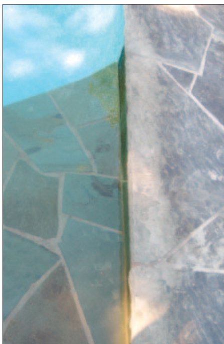
The damage done: Besides erosion on softer stone, some builders blame salt chlorination for grout dissolving out of joints (right) and concrete decks spalling (top). The problems seem to occur where wet and dry conditions exist, builders say, such as on the coping of this beach entry (bottom).
