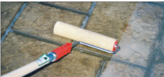
On deck: Topical sealers can be applied to new or old concrete, and most tile, by spraying or rolling the product onto the surface.
